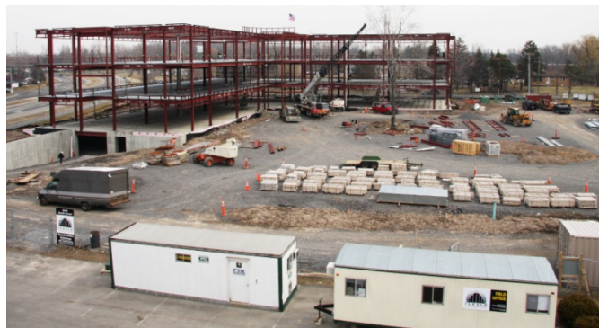
With the steel topping completed, workers now move on to the next phase of construction.
