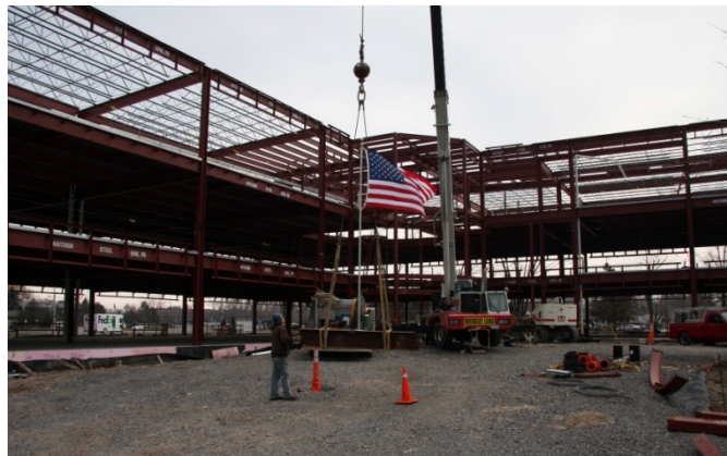
Workers begin to hoist the final piece of structural steel at 2410 North Forest.
