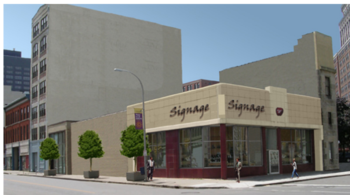
Iskalo Development is renovating the former Waldorf Lunch and Howard Shoes building at 5 East Huron
